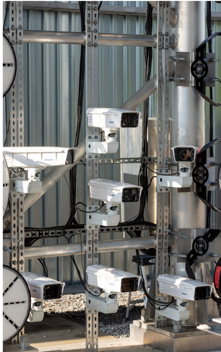
FIGURE 3. The cameras and lenses are installed inside protective enclosures and mounted on swing arms. (Courtesy of Norfolk Southern)
