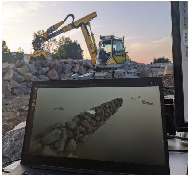
FIGURE 3. Computational planning and stone placement using the autonomous HEAP. (© Gramazio Kohler Research, ETH Zurich, Eberhard AG. Photo: Ryan Luke Johns)
