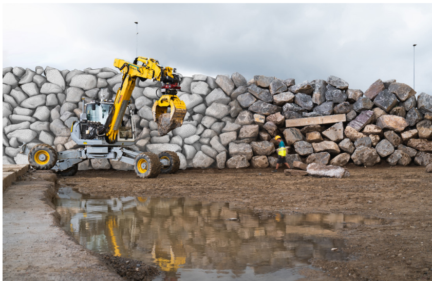
FIGURE 1. The Menzi Muck picked up and scanned each boulder as it built the wall. (Circularity Park in Oberglatt, Eberhard AG, 2021-2022 © Gramazio Kohler Research, ETH Zurich, Eberhard AG. Photo: Marc Schneider)
